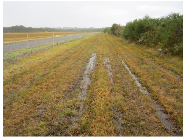
18/9/2015 - Grass access track on south side of grass runway. Water pooling in wheel tracks.
