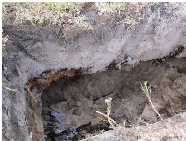
TP2 – Typical profile with aeolian sands, overlying a thin upper indurated sand horizon, overlying more aeolian sands where the test pit is collapsing due to water inflow occurring above a lower indurated sand layer.
